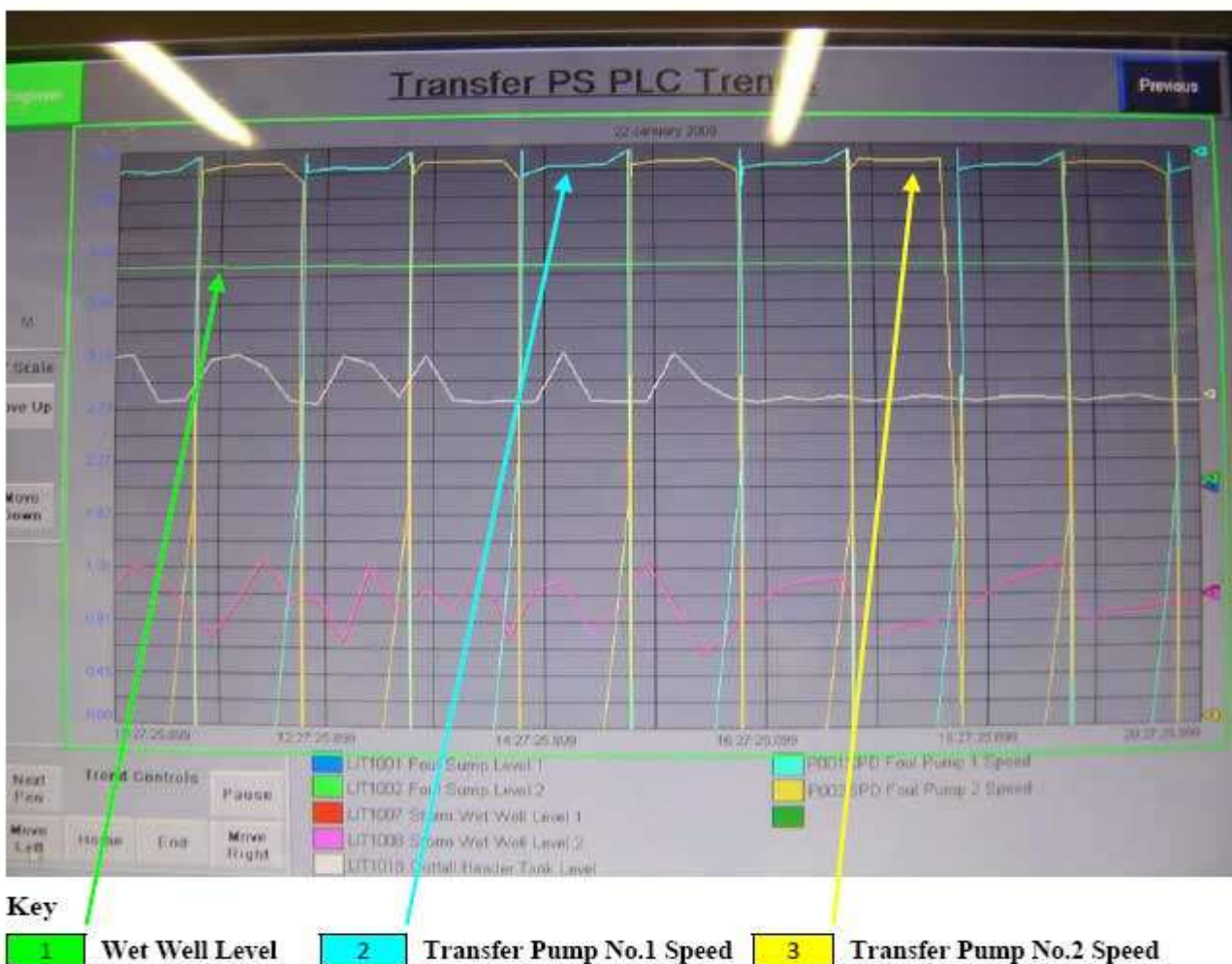
Figure 4.3.2.a – Details normal pump operation in times of high flow (and subsequent High Level).
