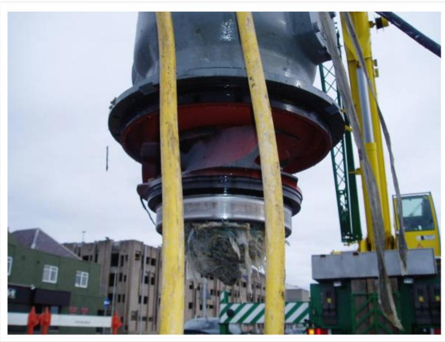
Typical Pump Blockage
